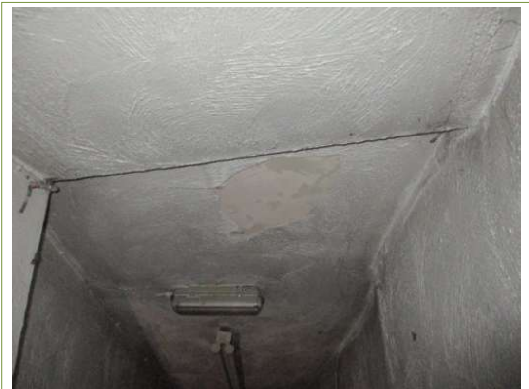
Textured floor coverings on the 1 st floor side stairwell ceiling. No ACM's detected
