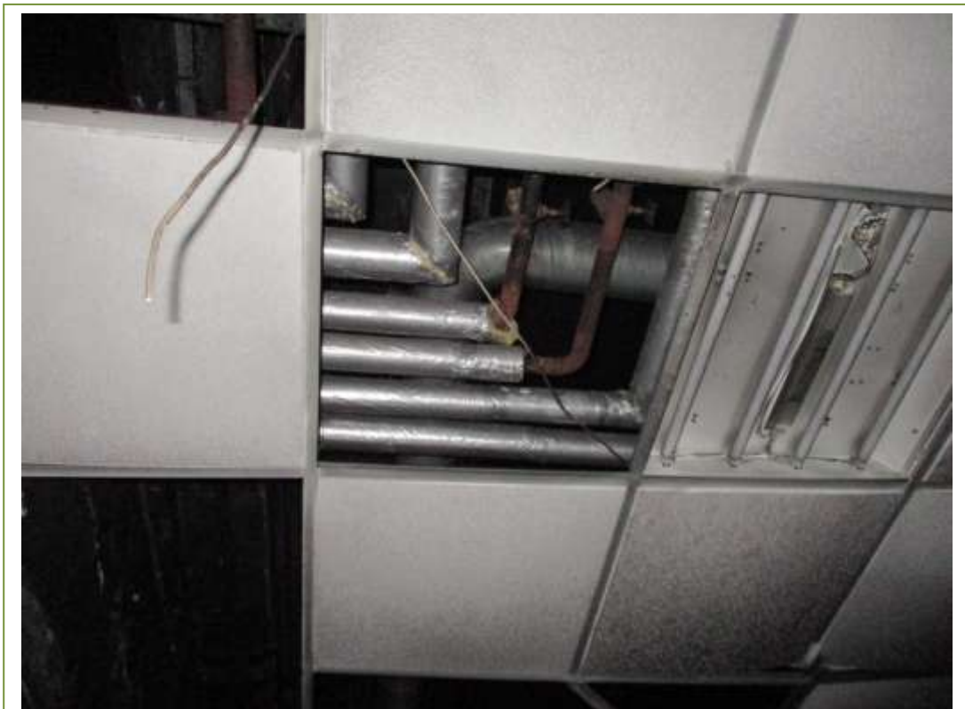
Fiberglass pipework insulation. No ACM's detected
